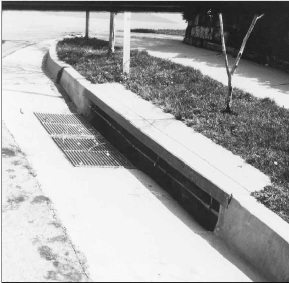
Figure 4-16. Sweeper combination inlet.
