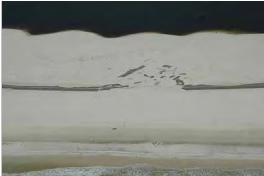
Figure 8.14. Pavement moved landward by overwash processes. (Gulf Islands National Seashore, Perdido Key, Florida after Hurricane Ivan; 2004).
