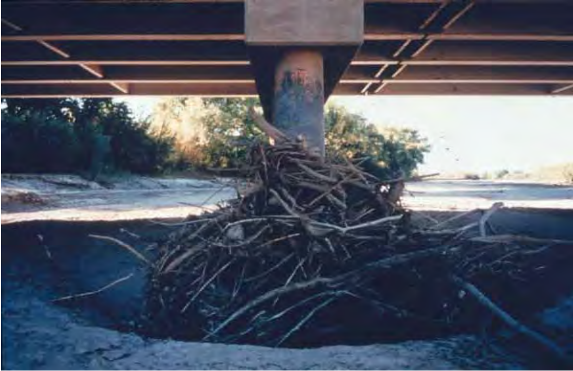
Figure 9.5. Scour at a Coastal Bridge Pier
