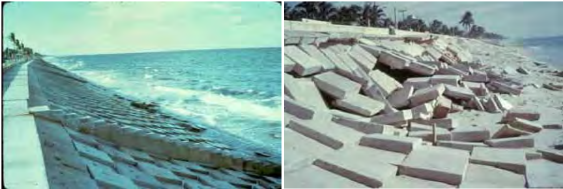
Figure 6.18. Example of rigid concrete-block revetment failure (Florida Highway A1A, Delray Beach, circa 1972; University of Florida and USACE archive photos)
