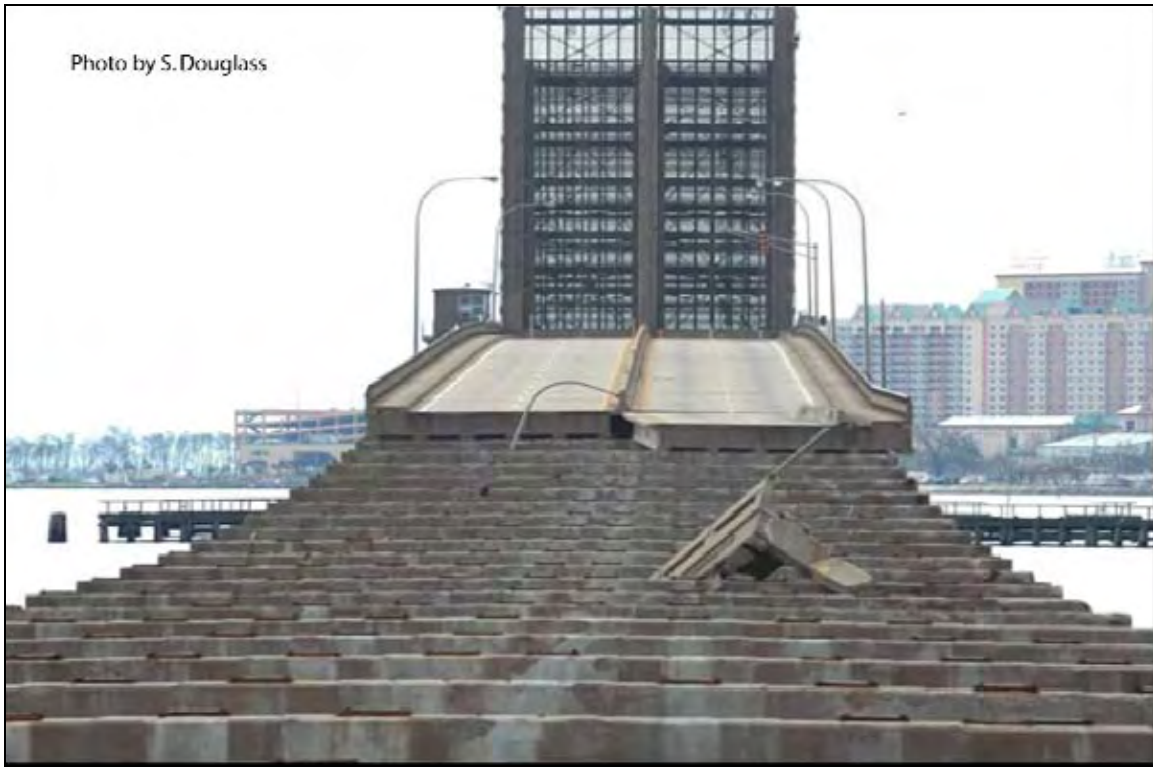
Figure 9.14. US 90 bridge over Biloxi Bay, Mississippi showing the spans at higher elevations were not removed (photo looking southwest from Ocean Springs 2/19/06.)
