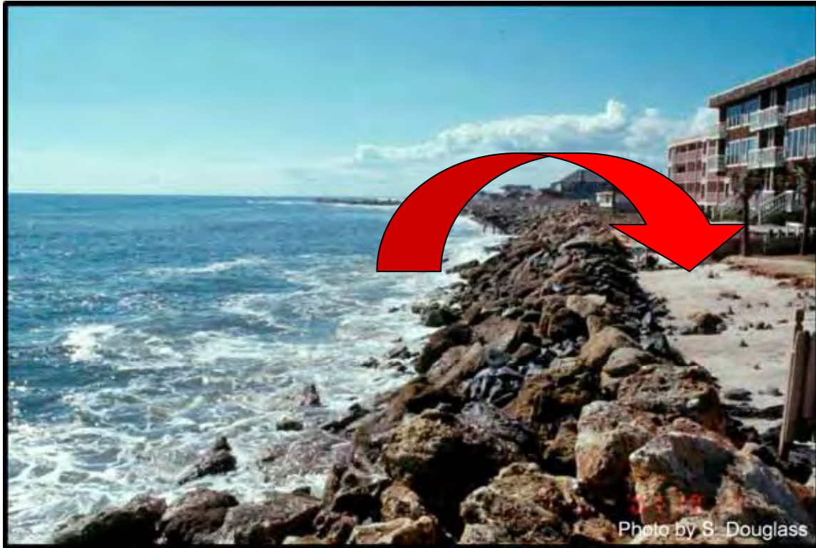
Figure 6.16. An example of splash damage behind seawall
