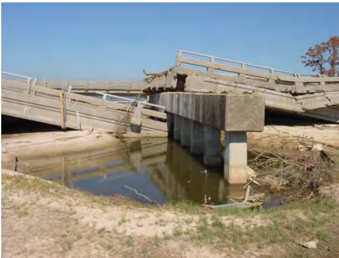
Figure 9.7. Wave scour hole formed by Hurricane Katrina.
