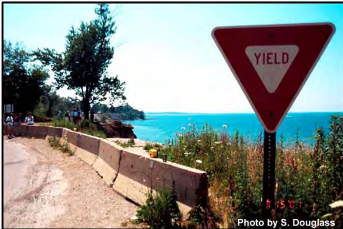
Figure 7.4. A local road being undermined by bluff erosion and long-term shoreline recession on the Great Lakes. Painesville, Ohio (2001)
