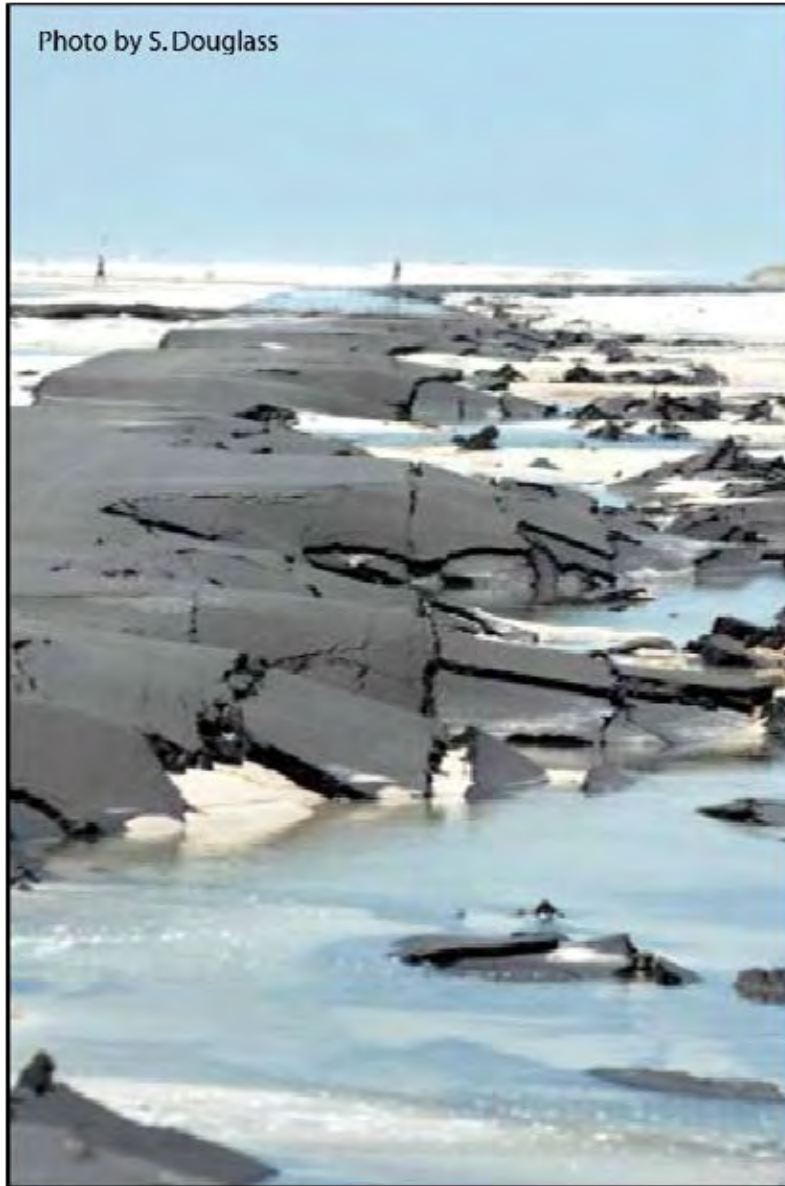
Figure 8.6. Pavement destroyed by the weir-flow mechanism (Ft. Pickens Road, Gulf Islands National Seashore, near Pensacola, Florida).
