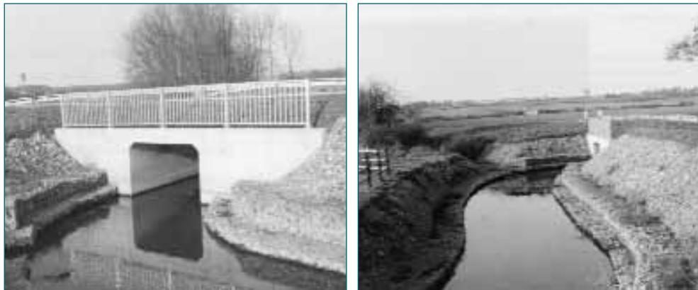
This culvert is not well aligned with the watercourse so the channel has been lined using gabions that both prevent erosion and help to improve the hydraulic conditions. Note the incoming channel on the left. Note also the use of the simple vertical headwall arrangement.
