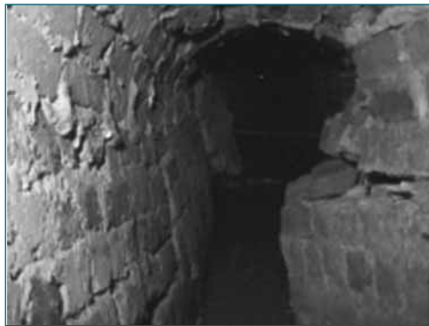
Figure A3.26 Inside the barrel of the culvert showing erosion to brick work and lateral movement of the RHS wall
