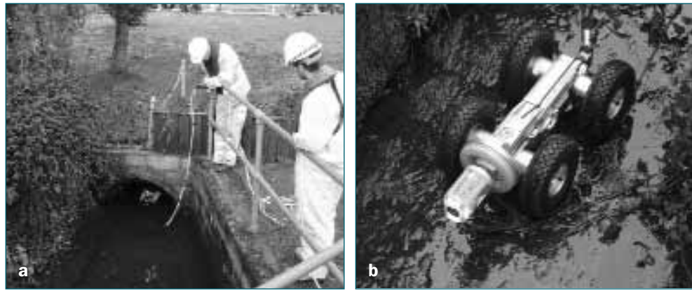
Figure 7.2 Culvert inspection using a CCTV system (a) and a typical tractor unit and CCTV camera (b) (courtesy Environment Agency and British Waterways)
