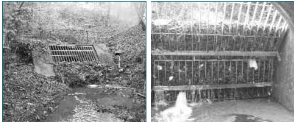
Figure 6.23 Screen with debris blinding (courtesy Transport Scotland)
