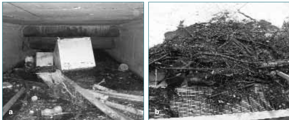
Figure 8.3 Obstructions within a culvert (a) and debris blocking a culvert entrance (b) (courtesy Richard Allitt and Scott Arthur)
