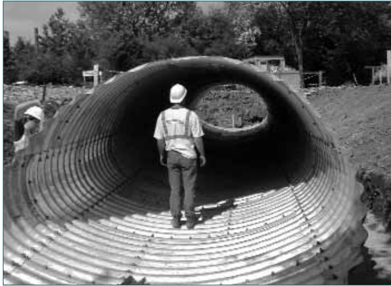
Note how the structure is formed from small panels bolted together on site.
