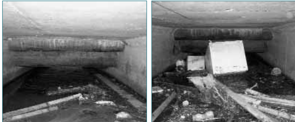
Two service pipes cross this culvert, significantly reducing its capacity and increasing the risk of blockage. Complete blockage could easily occur in a flood, causing severe flooding to local properties and infrastructure. Such blockages are difficult to remove and can only be cleared after the flood event. In the case of an existing situation such as this, the only solution may be to introduce a trash screen at the inlet, but it should be appreciated that this will impose a requirement for routine and emergency cleaning.
