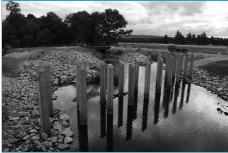
Note the timber screen posts are set into a low strength mortared socket, to allow future replacement. Suitable access for the removal of large pieces of debris is provided to the screen.
