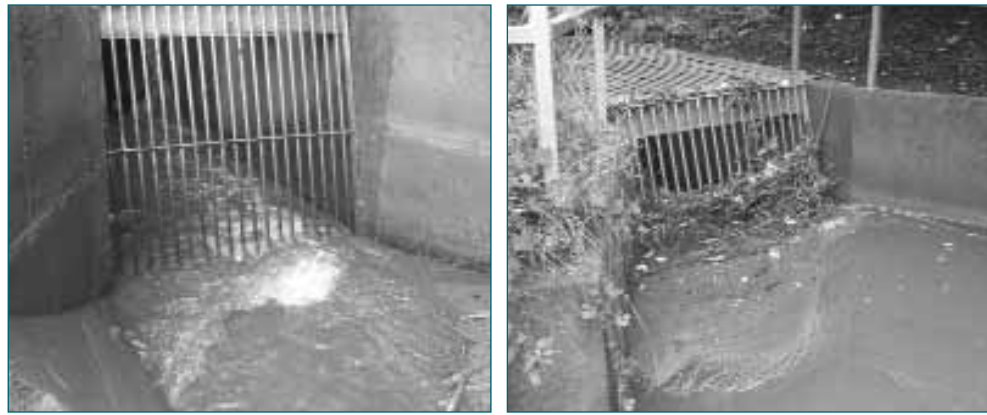
Figure 6.22 Clean screen and screen with partial blockage (courtesy Leeds City Council)
