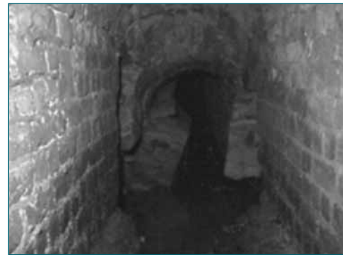
Figure A3.27 View showing lateral movement of sidewalls and partial collapse of roof element
