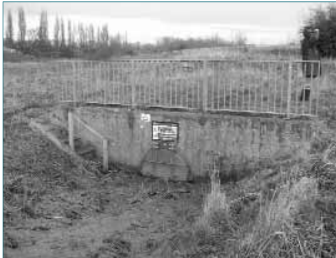
Note: The effective operation of this outfall has been compromised by the condition of the channel downstream. The flap gate should be free to open under the pressure of the water in the culvert.
