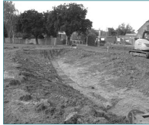
Figure A3.37 Final removal of existing culvert and preparation of new channel bed (courtesy Andy Pepper)
