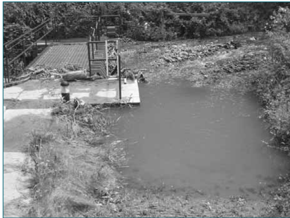
Figure A3.41 River Jordan debris screen following high-flow event in June 2007. Note that debris has accumulated upstream of the screen up to the level of the cleaning platform (courtesy Environment Agency)
