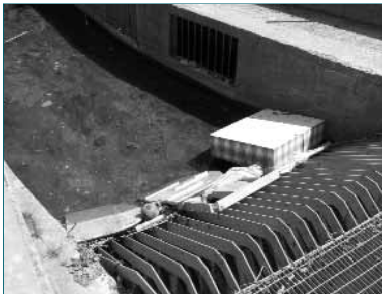
In this case the urban debris has been prevented from entering the culvert by the screen. This type of material could readily block a culvert with severe consequences. Note that there is a bypass facility at this screen to carry flood flows if the main screen is partially blocked by debris.
