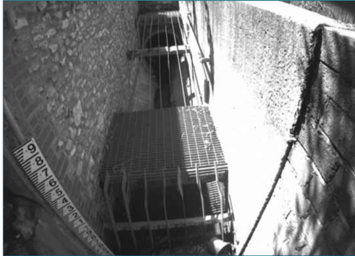
Figure A3.7 Kennaway screen looking upstream
