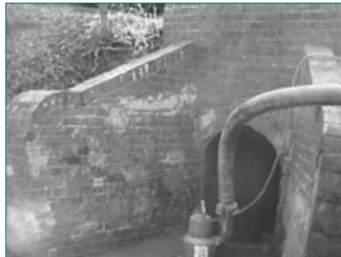
Figure A3.24 Entrance to the culvert, showing large angled brick wingwalls and brick headwall. A pump was used to enable works to be carried out
