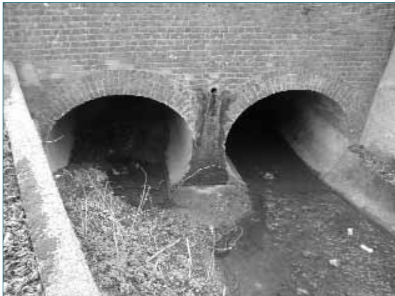
At this culvert the channel upstream is aligned with the right-hand barrel and sediment has been deposited in the slack water area upstream of the left barrel. The left barrel has significant sediment deposits, reducing its capacity. A small amount of sediment in the left barrel might be acceptable (the determination of what is acceptable would be part of the performance assessment process), and would provide a dry route for wildlife migration in low-flow conditions, but in this case the sedimentation was excessive and had to be removed.
