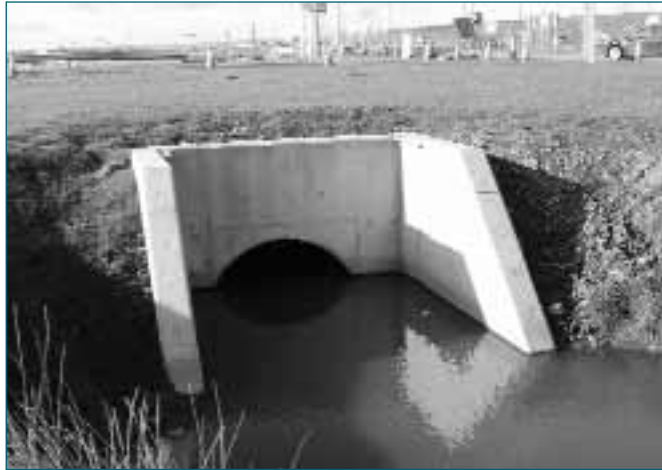
Figure 7.5 Culvert where normal levels would prevent access for inspection (courtesy Transport Scotland)
