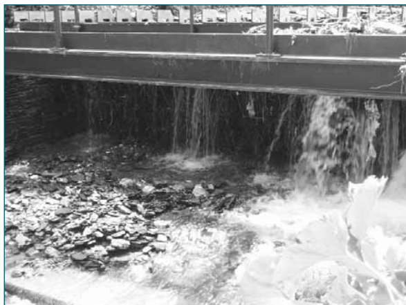
Figure A3.42 River Jordan debris screen following high-flow event in June 2007 (courtesy Environment Agency)
