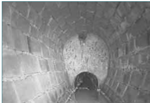
Figure 7.3 A typical still image from a CCTV survey, showing a change in section of a pipe (courtesy Richard Allitt)
