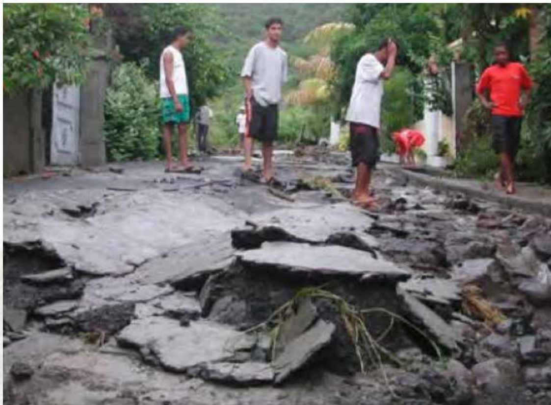
Road damaged due to torrential rains
