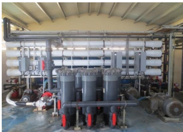
Figure 3.2 Desalination Plant at Anse aux Anglais. Credit: MoESDDBM
