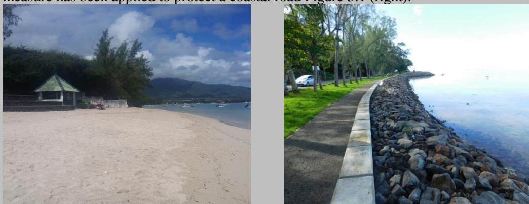
Figure 5.1: (left) Beach nourishment at La Preneuse and (right) Rock revetment for shoreline protection at Baie-du-Cap (Source: MoESDDBM)
