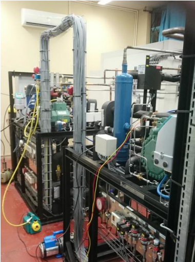
Figure C.1 Equipment at UDM for a pilot study
