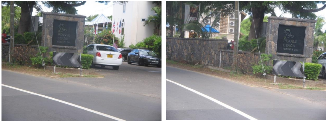
Figure 7.2: Photographs of Damaged Directional Road Sign
