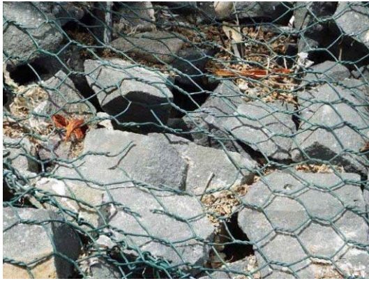
Damaged gabion walls
