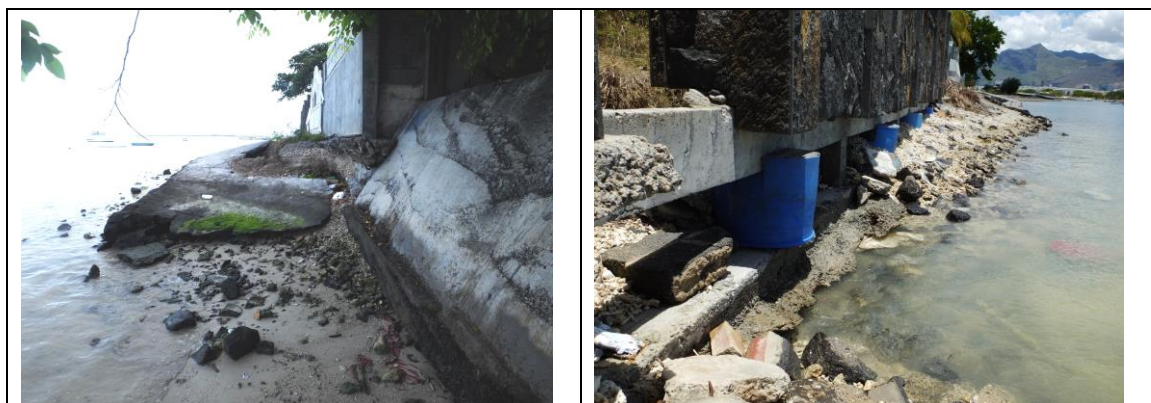
Figure 3- Eroded Coastline and Boundary Walls
