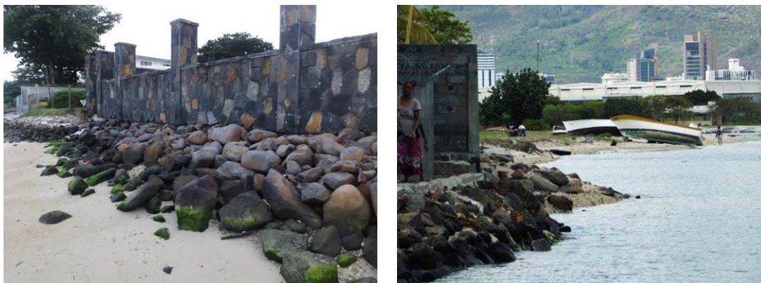
Eroded narrow beach at N end
