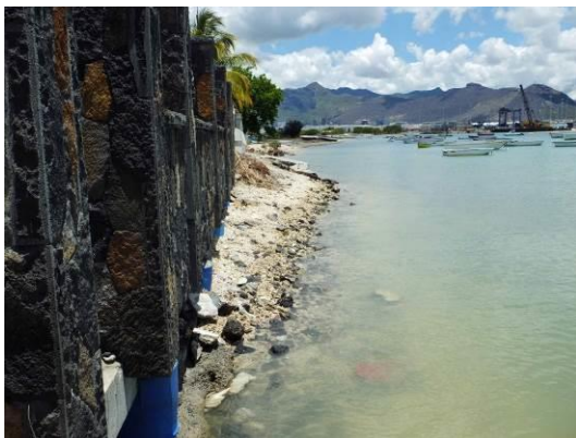
Hazardous pedestrian access
