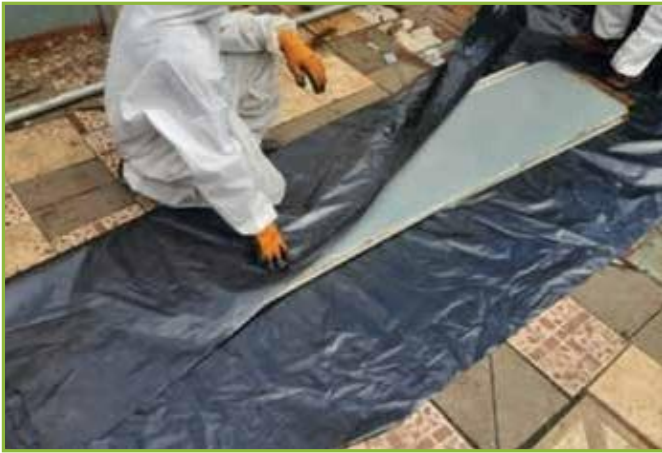
Figure 23: Wrapping of Asbestos sheets in polyethylene sheets prior to carting away to the landfill
